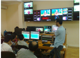
Police TV - Master Control Room
