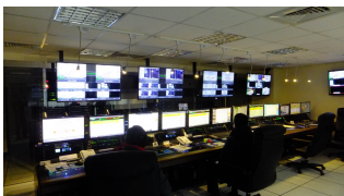
MOMO master control room
