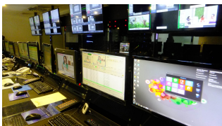
MOMO master control room
